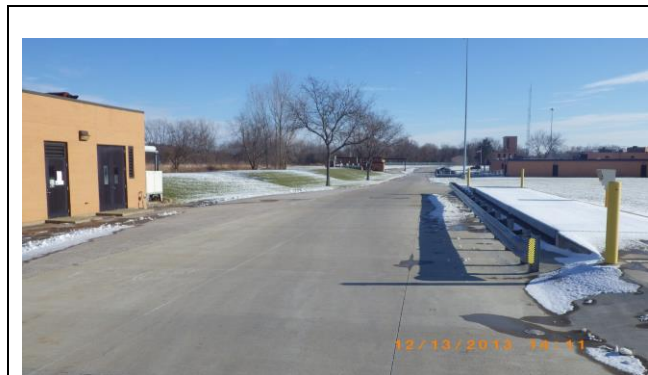
Typical storm sewer catch basin located within paved areas.
