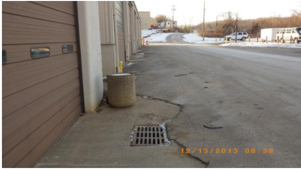
Typical storm sewer catch basin located within paved areas.
