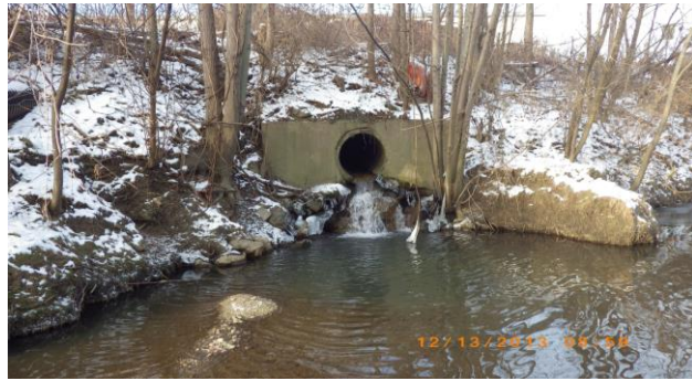
Dry weather flows from Outfall 002 were noted during the site inspection.
