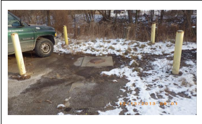
Oil/Water Separator located east of the service complex.
